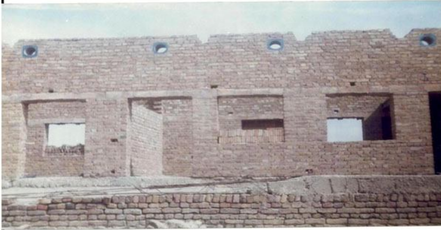
Incomplete building of Madrassah Arabia Dar ul Uloom Karimia
